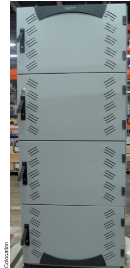
Colocation 19" enclosure Enclosure separated in 4 parts to give different access to each customer. Each hosted customer has his own secured access and cannot make some operation to the other part of the enclosure
