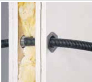
Wall feed-through in plaster-board fire-protection wall.
