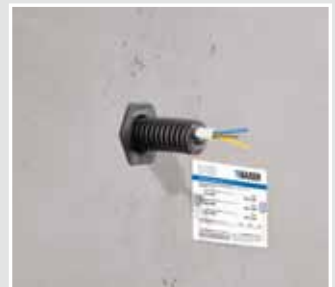
Wall feed-through in concrete fire-protection wall.
