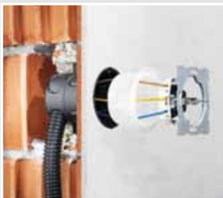
Later air-tight closing of flush-mounting boxes.
