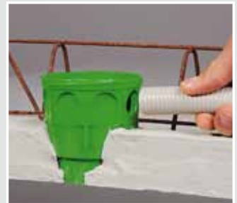
The conduit is inserted tightly and accurately and the box is sealed with the cover.
