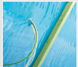
The cables are fed through the building's air-tight seal. This entry must be permanently sealed air-tight.
