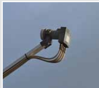
4 coaxial cables are connected here for reception.
