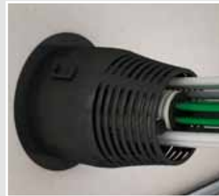
Mixing of cables and conduits.
