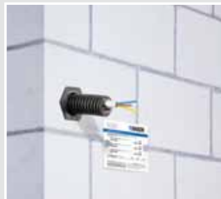
Wall feed-through in sand-lime brick fire-protection wall.
