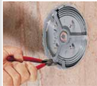
After removing the formwork: remove the bridges and open the front part.
